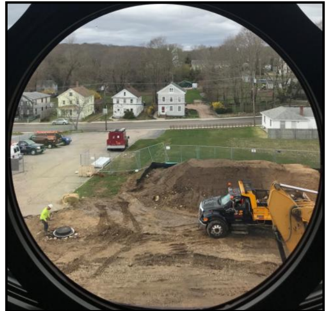
The construction site in July through a transept window of the church.
