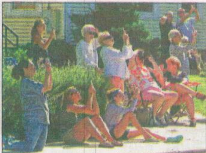
Spectators across the street in front of St. Michael School had cameras in hand as the steeple was lifted into place.
