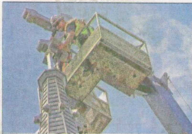
Matthew Gay, right, and Barry Antle, from steeple-maker Campbellsville Industries, use a crane bucket to delicately place the cross atop the steeple's spire.
