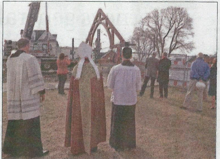
The raising of the first roof truss marks a milestone in the $8 million project to rebuild St. Michael's Church, replacing the original structure that was built in 1861.
