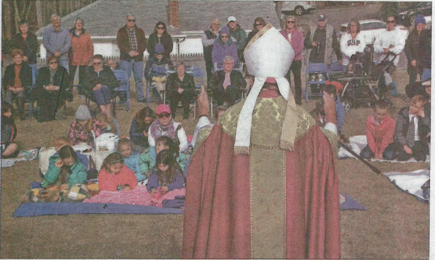
Bishop Michael R. Cote, of the Roman Catholic Diocese of Norwich, addresses the crowd prior to the blessing of trusses and the raising ceremony. The St. Michael's the Archangel Church community gathered to watch as Bishop Cote blessed the timber trusses Monday morning and to witness the first truss being raised for the parish's new church. Vermont Timber Works has been on site assembling the roof trusses for the last couple weeks in preparation for the event, a significant step in the church's reconstruction.
