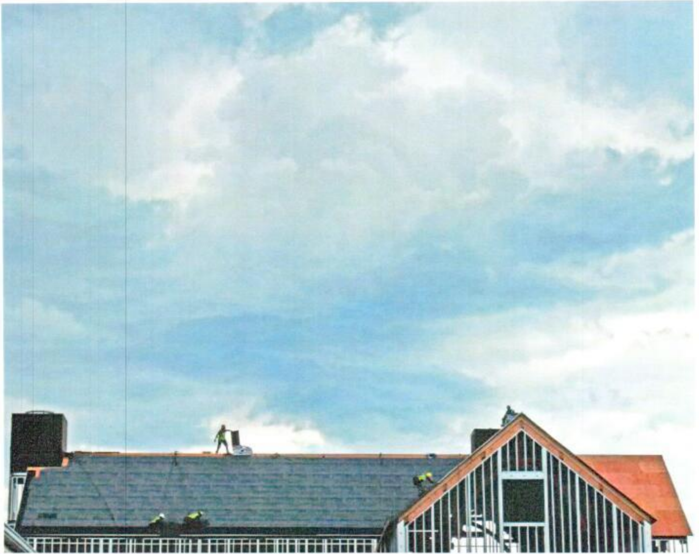
Under stormy skies and occasional showers, workers with safety harnesses began the task of shingling the huge roof of the new St. Michael the Archangel church building in Pawcatuck on Tuesday, June 27, 2017. | Harold Hanka, The Westerly Sun
